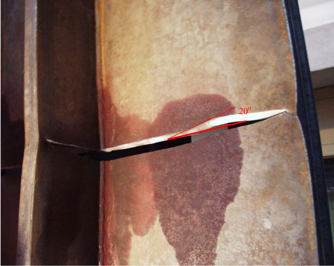
Figure 3-15 Final crack length and crack turning
