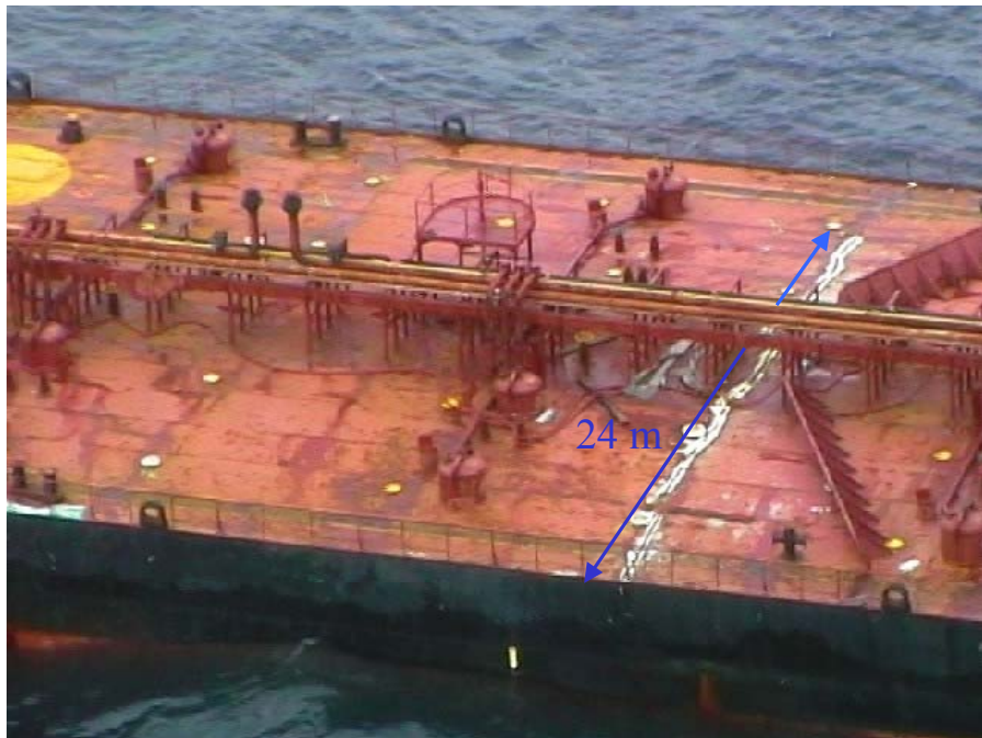
Figure 1-1 Cracked deck in the tanker Castor [1]
