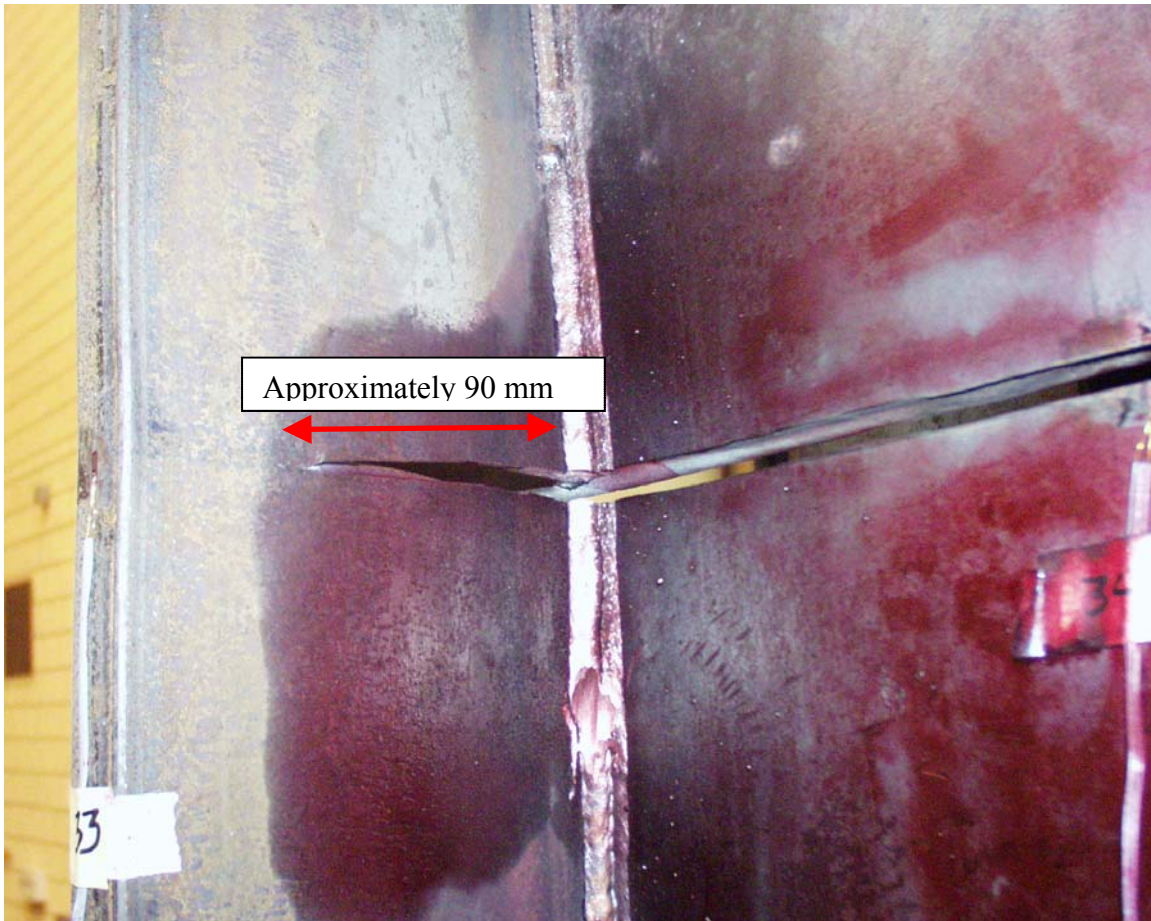
Figure 3-9 Crack propagation for S1 in the plate and the second stiffener (South side)
