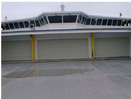
Forward Roller Doors
