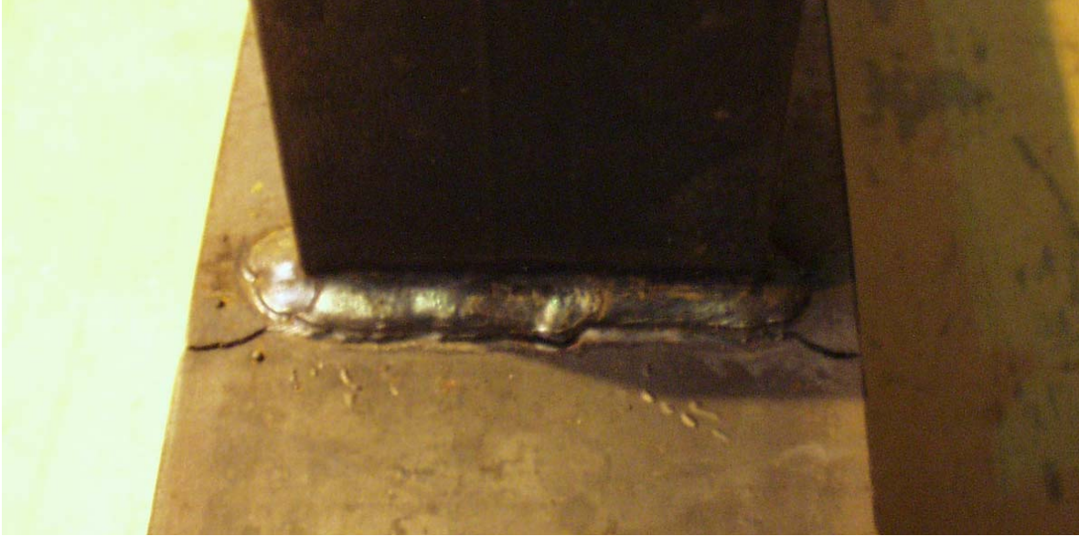
(a) Crack along beam flange
