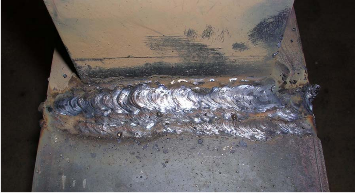
(a) Repair of attachment side of beam flange, Specimen C at flange of Tee 4
