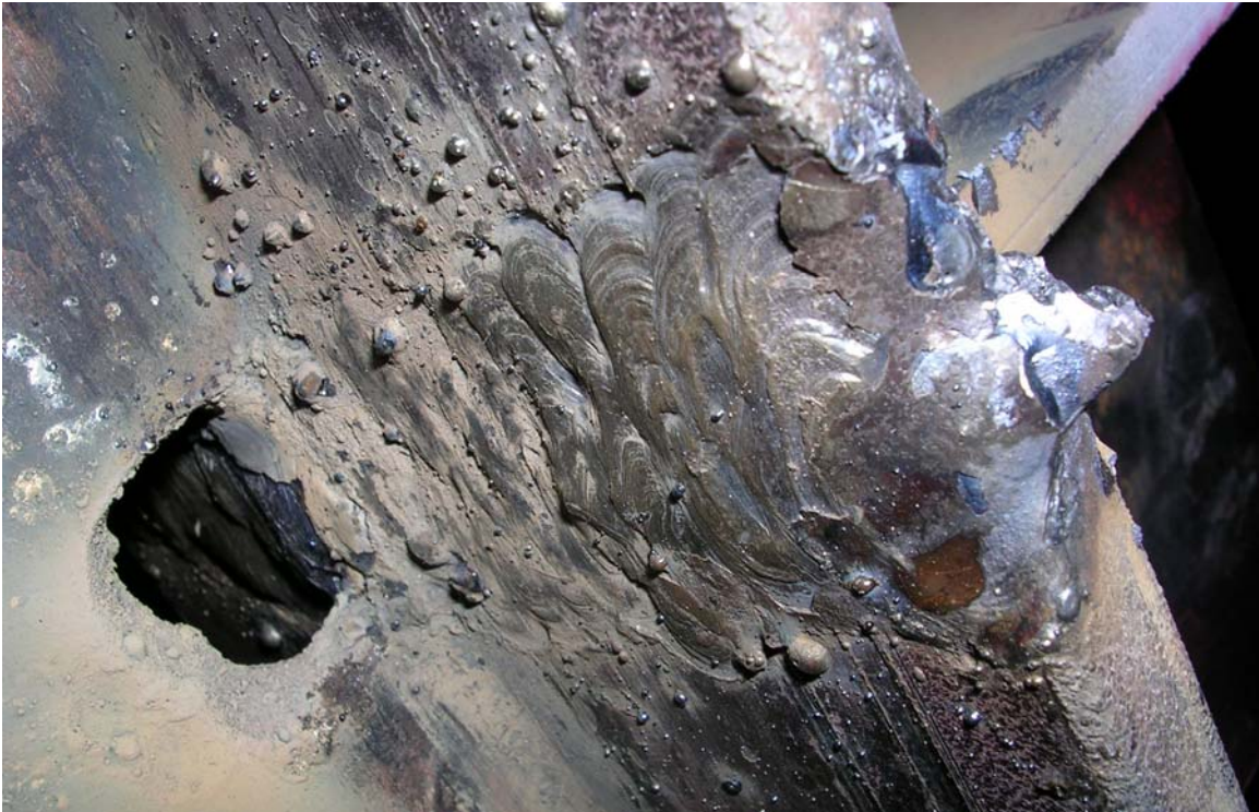
(b) Repair of web side of beam flange, Specimen C at flange of Tee 4
