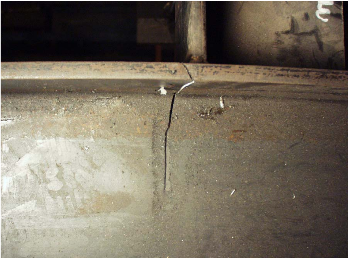
(b) Crack in beam web
