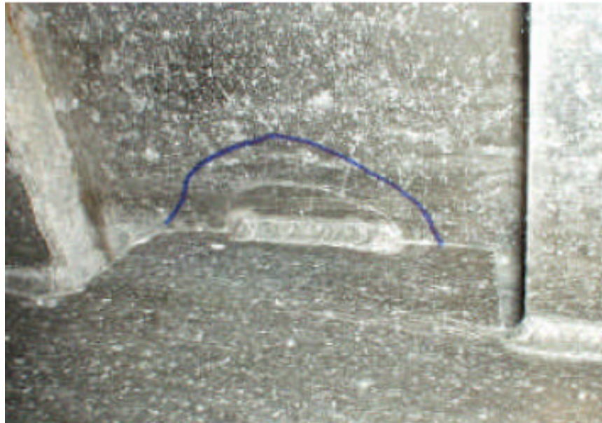
An example of intergranular corrosion (Bushfield et al., 2003).
