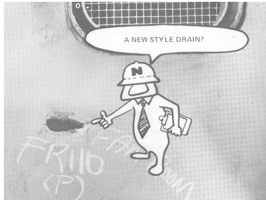
Figure 12-3: Corrosion where standing water at an internal stiffener permitted buildup of salt concentrations (Dye and Dawson, 1973).
