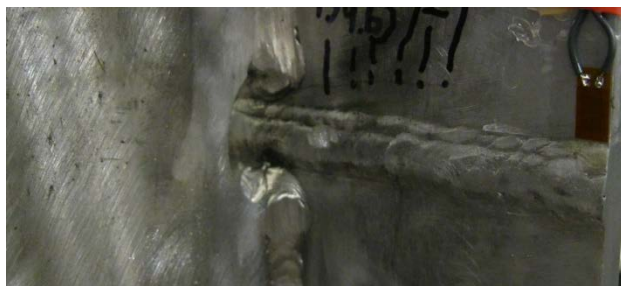
Figure 2. The butt weld and rathole where crack initiation occurs are displayed.
