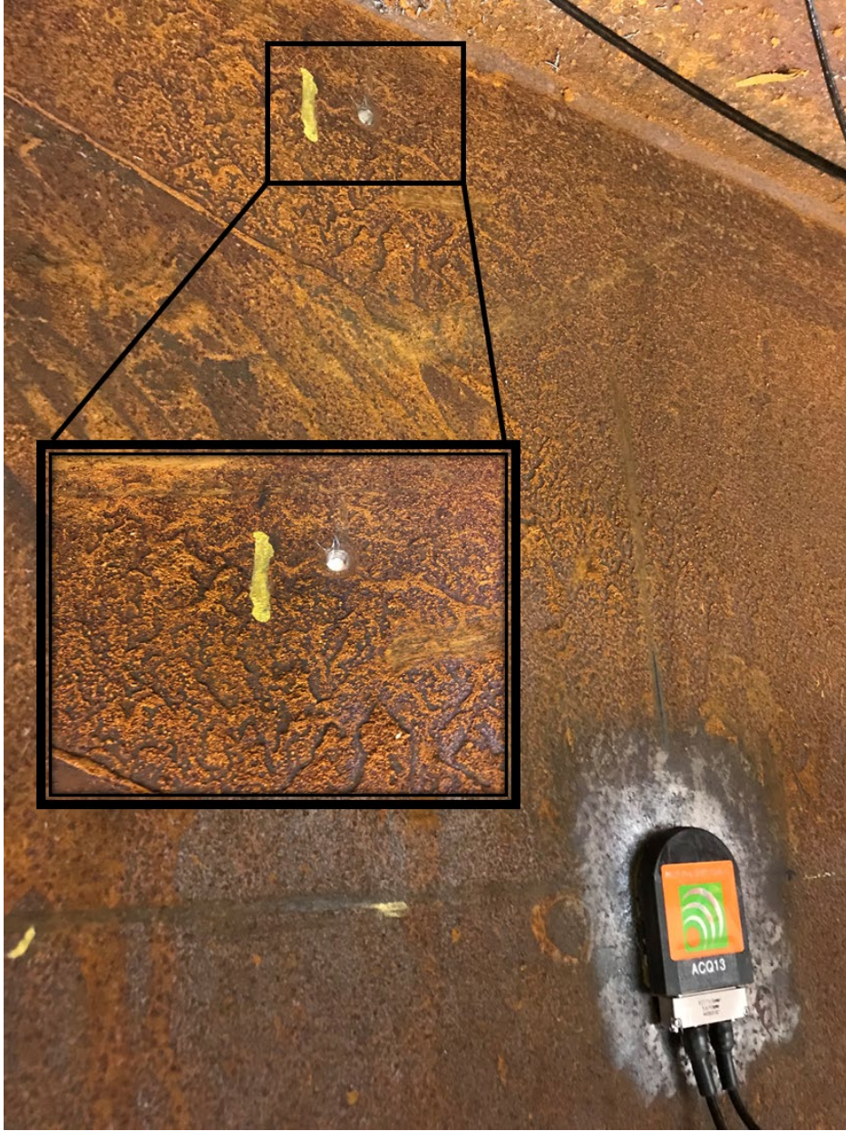
Figure 14. Damage 1, a 1/4-inch through-hole, shown in relation to ACQ 13
