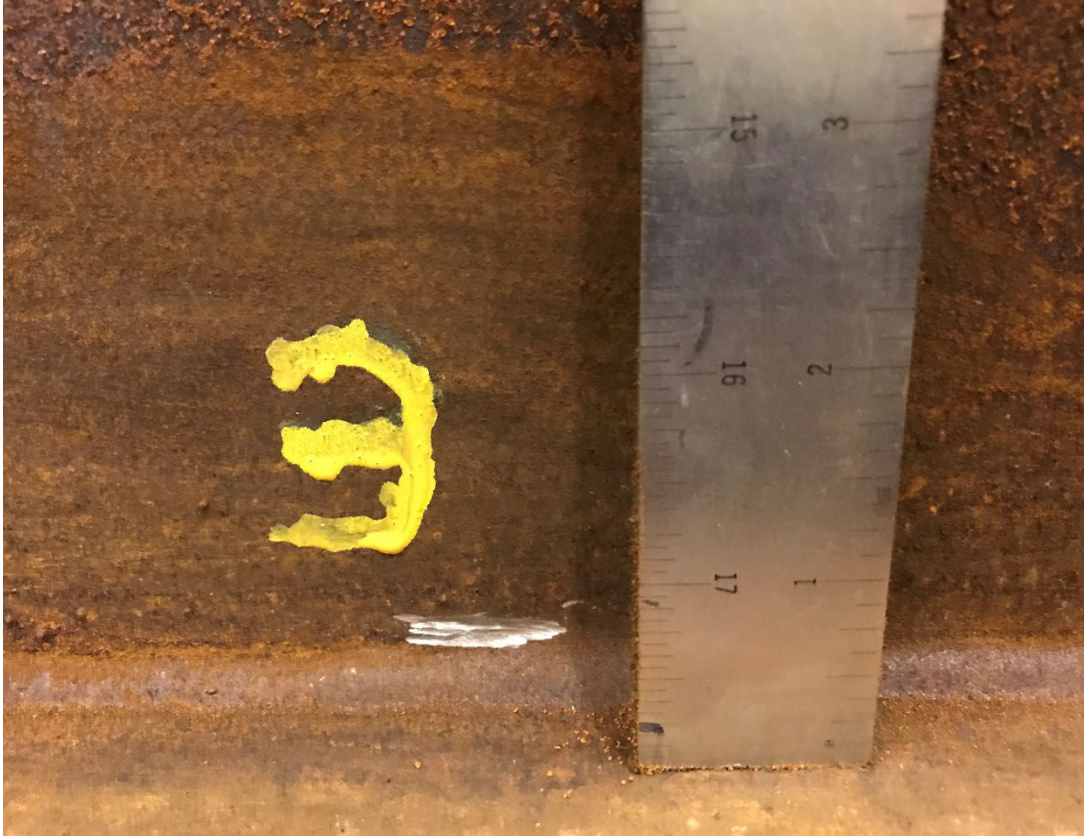
Figure 15. Damage 3, a simulated crack at a longitudinal stiffener weld toe
