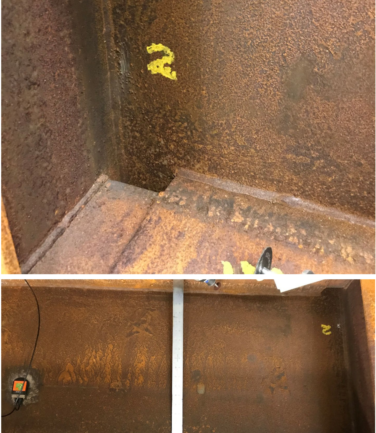
Figure 53. Damage 2, a simulated transverse stiffener weld toe crack (top) and its relation to ACQ 13 (bottom)
