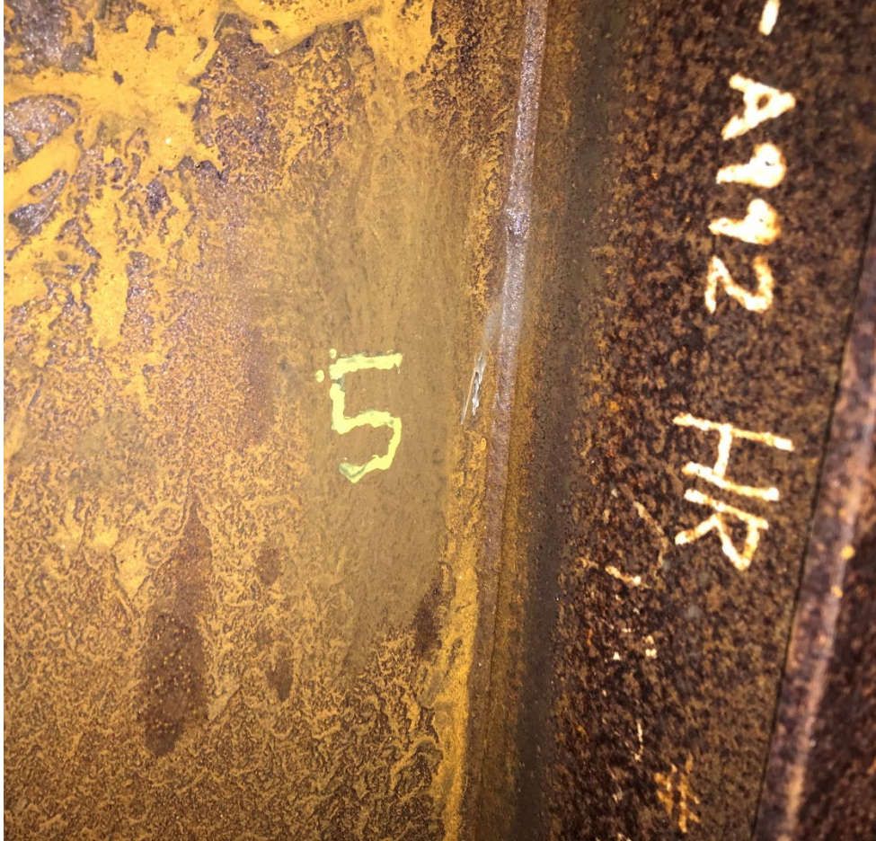
Figure 55. Damage 5, a simulated transverse stiffener weld toe crack
