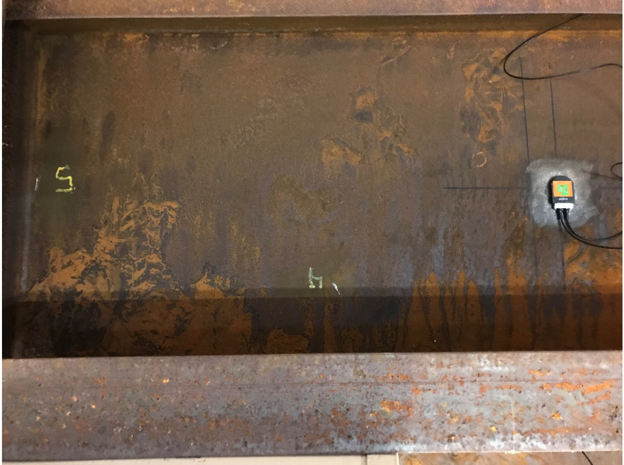
Figure 56. Damage 4 and Damage 5 in relation to ACQ 14
