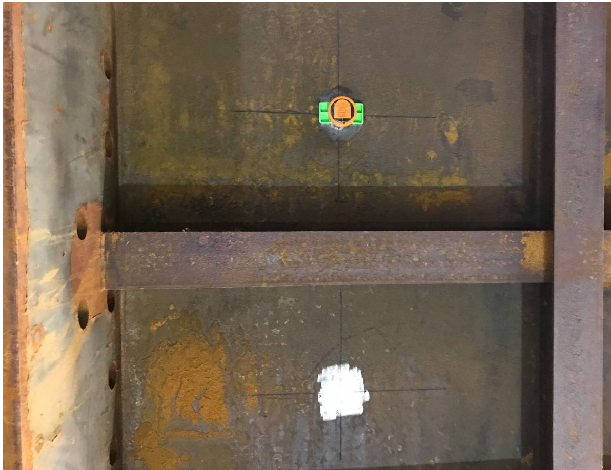
Figure 5. Sensor installation tool holding the sensor base for ACQ 11 in place for the cure cycle (top) and area marked and prepared for installation of ACQ 12 (bottom)
