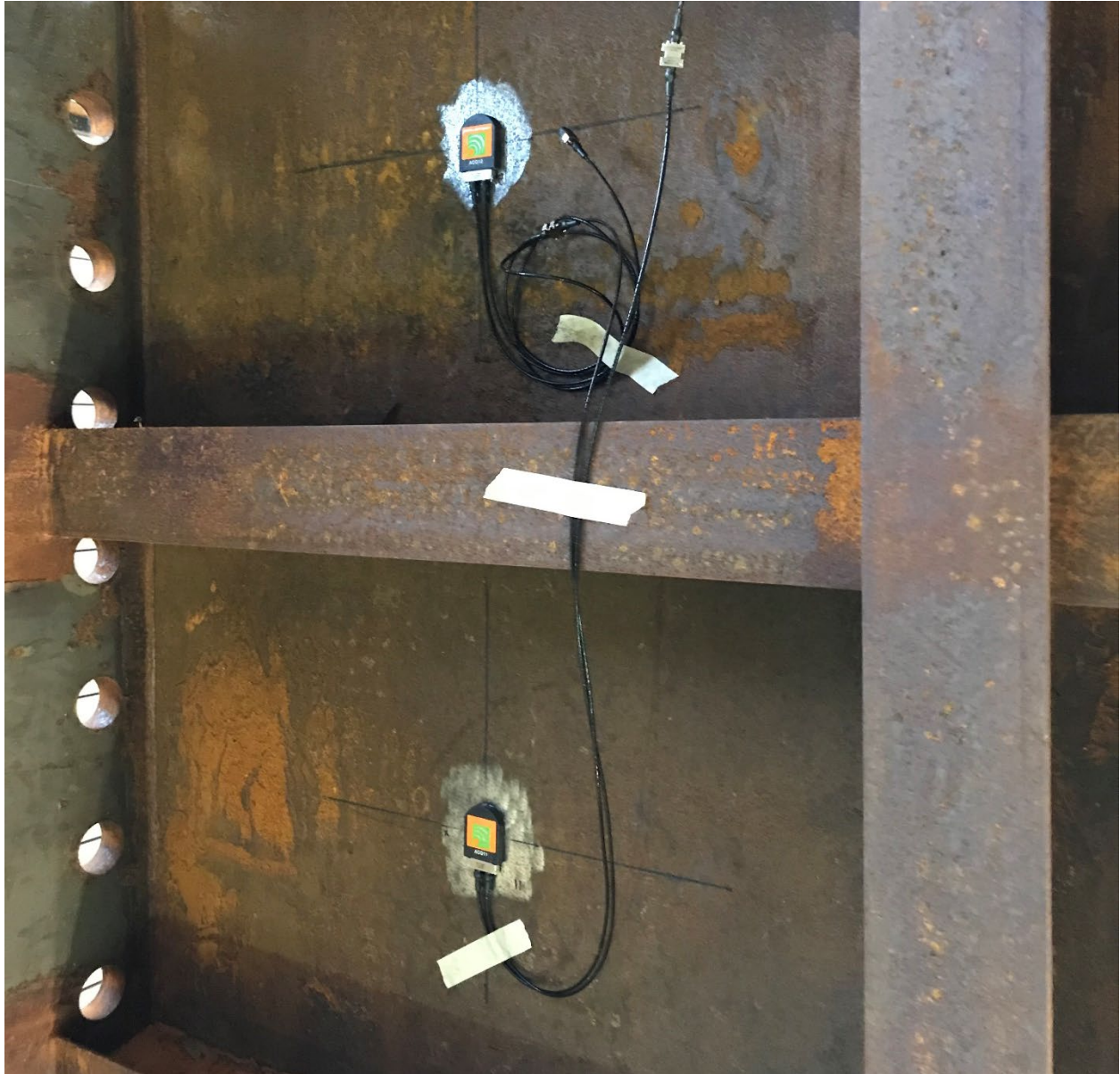
Figure 6. ACQ 11 (bottom) and ACQ 12 attached to the sensor bases with cables installed
