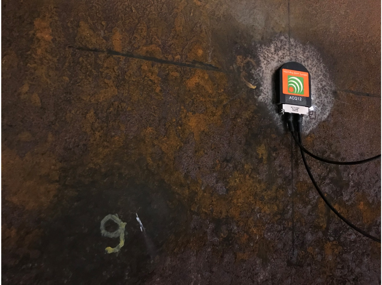
Figure 57. Damage 6, a simulated plate crack, in relation to ACQ 12
